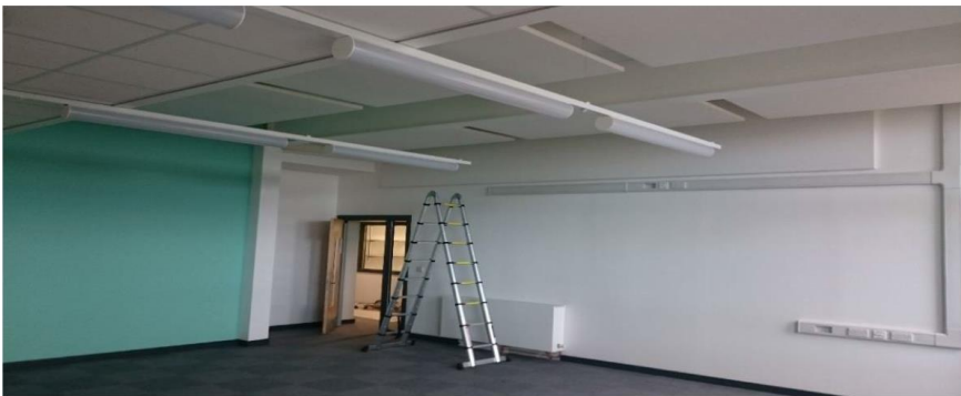
Figure 4: Primary school classroom. The underside of the bulkhead can be seen in the foreground, top left of the picture.
